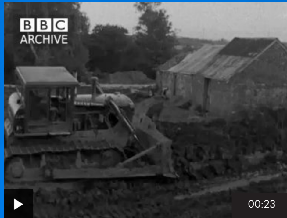
M1 Motorway, Diggers working around a solitary house From: "Completion of M1 delayed by presence of single house" (1966)
