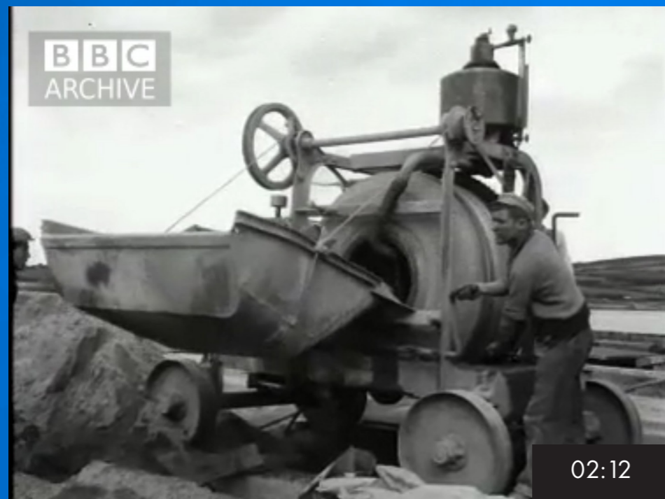
Shows the construction of a new pier in Larne, County Antrim to increase the size of the harbour. From: "News: New Pier for Ulster" (1954)
