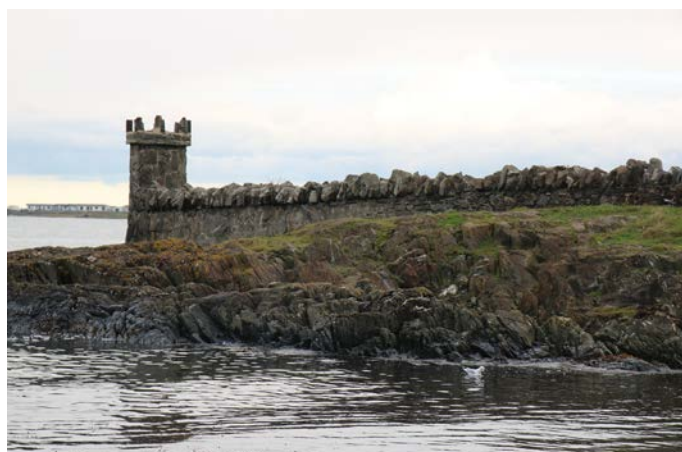
"Shore at seawall 2"
